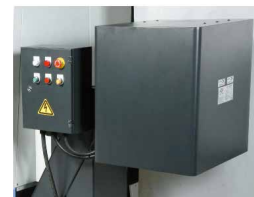
The motor of the chip remover stops and turns off
