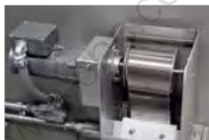
Oily water separating installation
